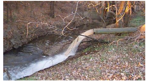
DEQ file photo of a point source discharge
